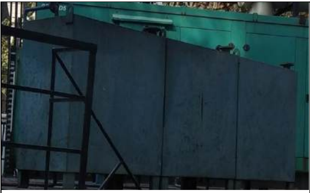
Diesel storage tank for DG set
